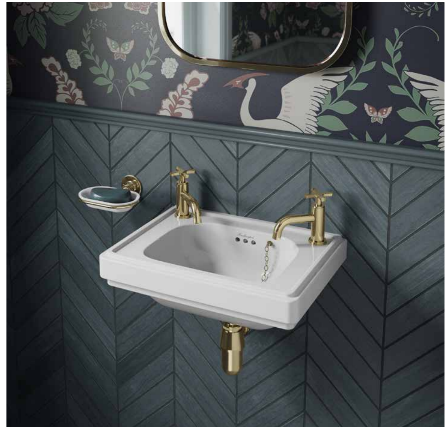
Riviera 450mm 2 tap hole cloakroom basin, Riviera pillar taps, plug and chain waste and bottle trap. Soap dish and Towel ring. Riviera back-to-wall WC with soft-close seat, concealed cistern including lever. WC roll holder. All fittings and accessories are Gold finish.
